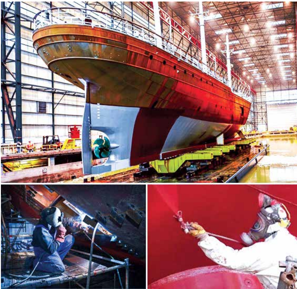
Crafting Maritime Excellence: Skilled workers in the shipbuilding and repair yards of Bangladesh diligently ply their trade, demonstrating expertise and dedication as they construct and refurbish vessels, contributing to the growth of the nation's maritime industry
